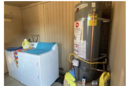
shed laundry water heater
